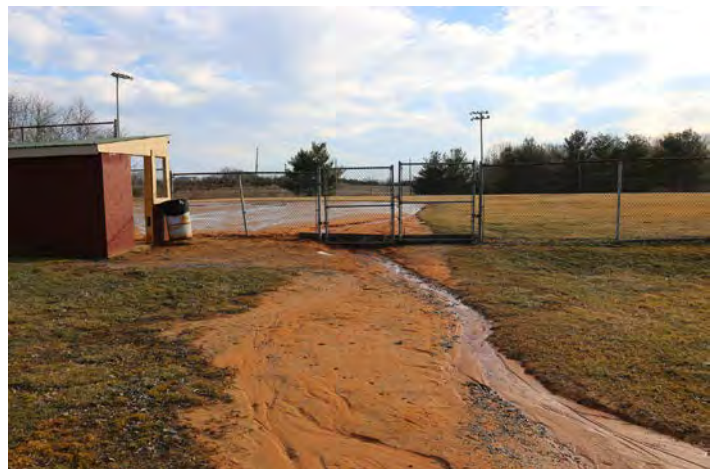
Ballfield - Note poor drainage.
