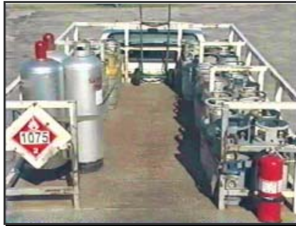
Figure 5.1.6b – Vertically Secured Cylinders
