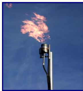
Figure 5.1.8d – Propane Burning from Flare Tower
