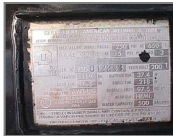
Figure 5.1.7d – Underground Tank Data Plate
