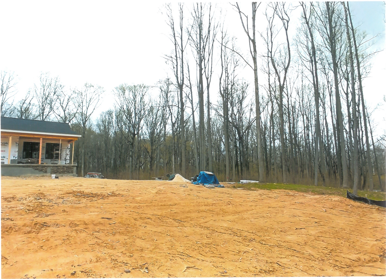
Rock break, tree line near (N) house
