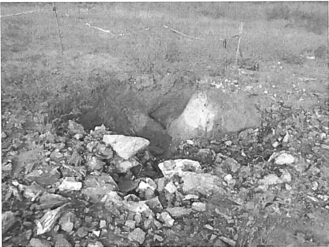
Sinkhole in basin #2.
