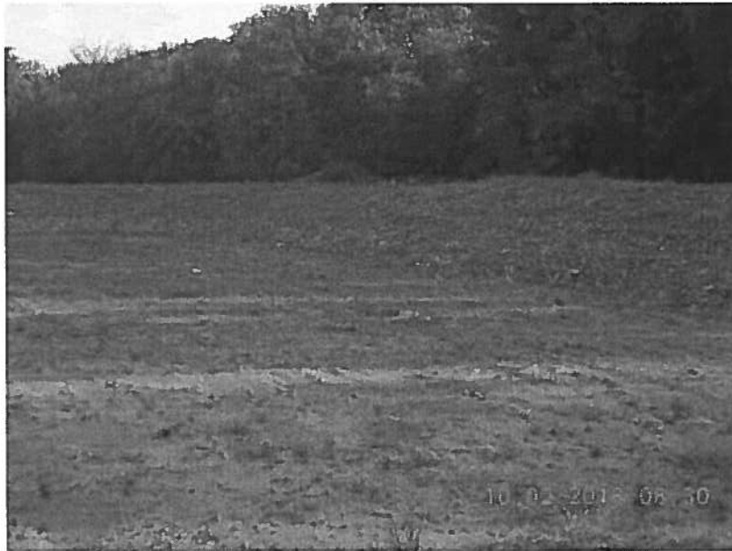
Fifth potential sinkhole pictured in the reuse pond.
