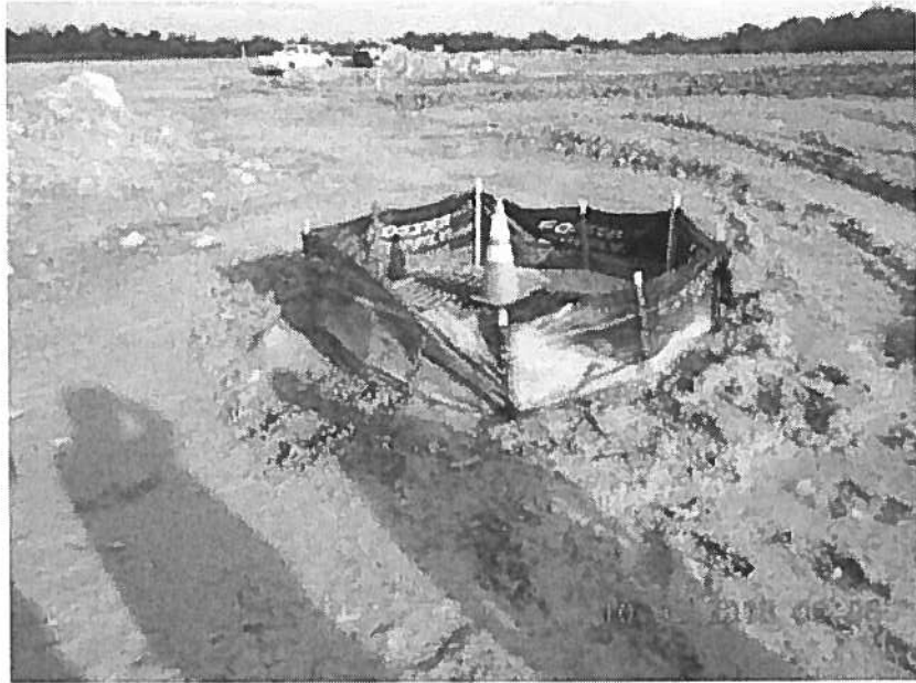
Sinkhole # 7 capped under concrete drop inlet structure.
