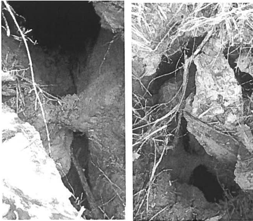
Sinkholes – Rt. 9 Bike Path, Kearneysville to Coast Guard Roads, March 2019, (Photos: T. Cannon)
