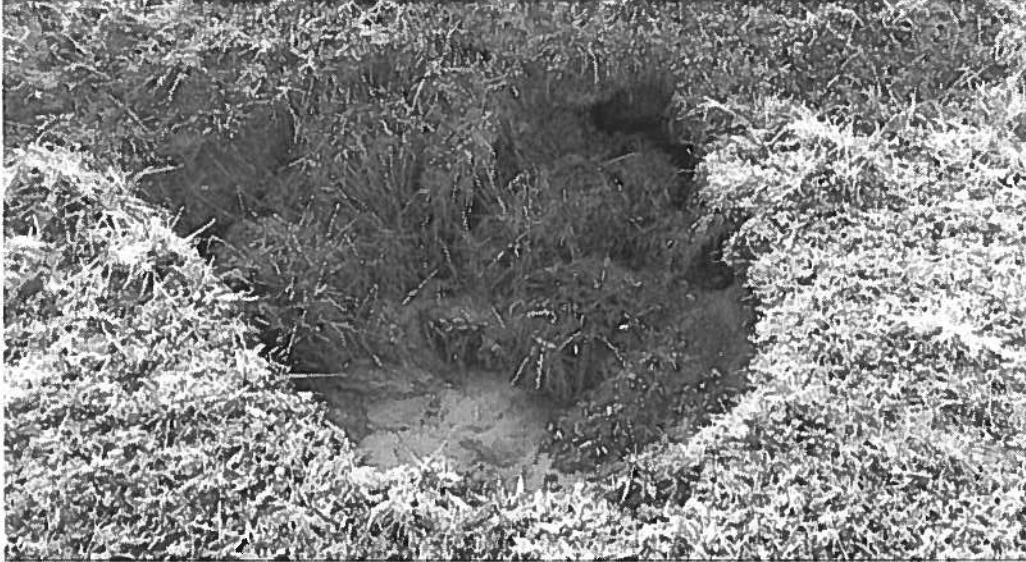
Sinkholes - Rt. 9 Bike path between Northport Ave., Kearneysville (Photos; S. Writ)
