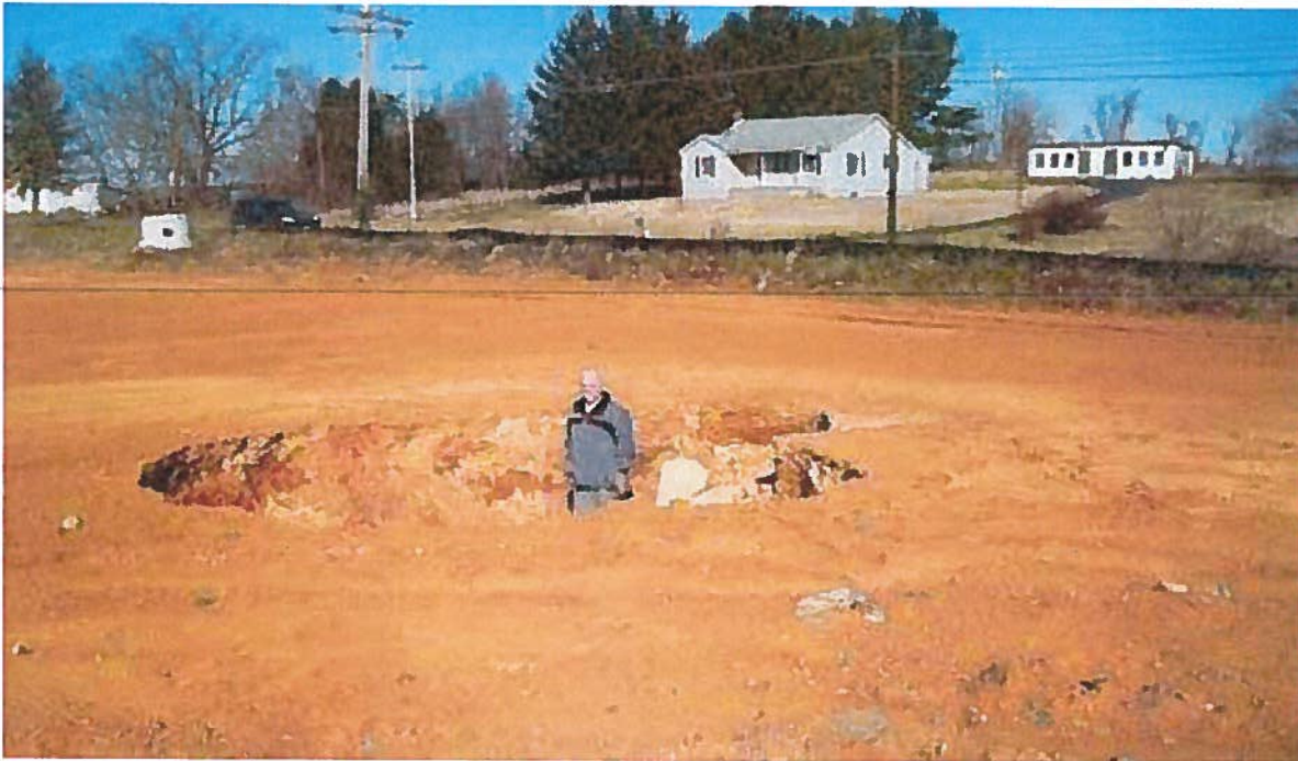
(Sinkhole at the abandoned Tackley Mills subdivision at the intersection of Old 9 and Wiltshire Bld. The sinkhole grew large enough to threaten Old 9)
