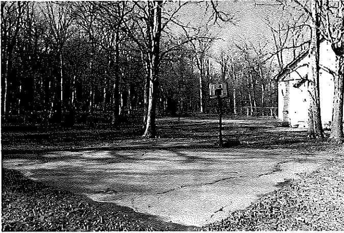
Half court basketball - Note condition of court surface.
