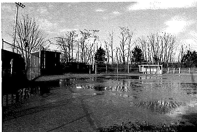
Ballfield - Note poor drainage.
