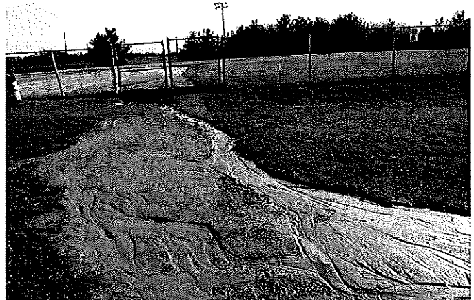
There are fundamental infrastructure improvements needed throughout the Jefferson County parks.
