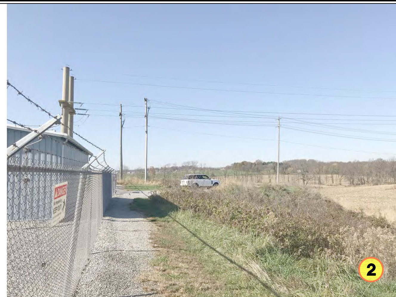
View west near balloon tether at northeast corner of substation, looking along northern fence
