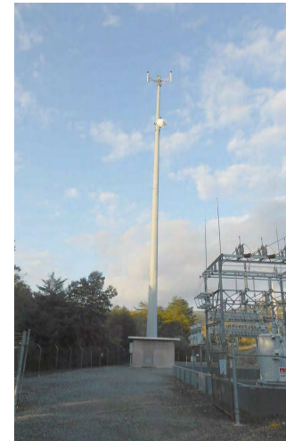
TYPICAL MONOPOLE PHOTOGRAPH NO SCALE
