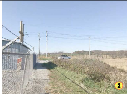
View west near balloon tether at northeast corner of substation, looking along northern fence
