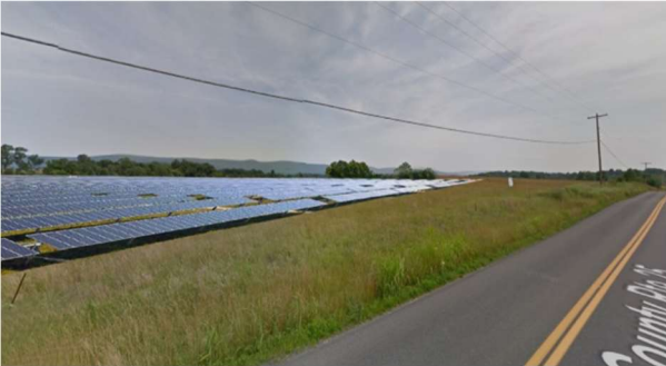
Unscreened Solar Panels
