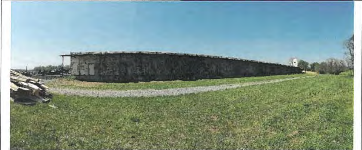
Image 9. Southeast side of the building (which faces the railroad tracks) from south corner.
