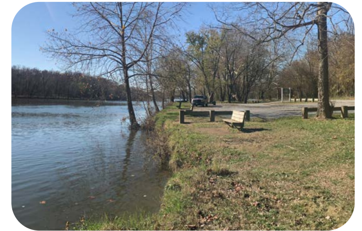
Photo of Erosion on at existing riverfront park from GoogleMaps
