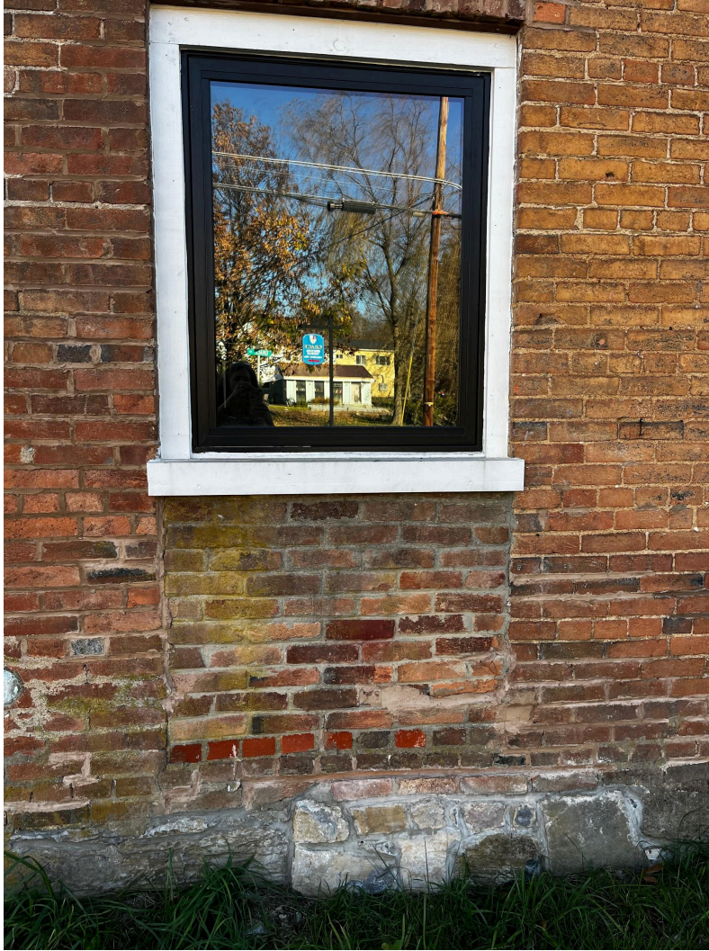
This is an example of mismatched bricks after the structure was hit by a vehicle. (Middleway, WV)
