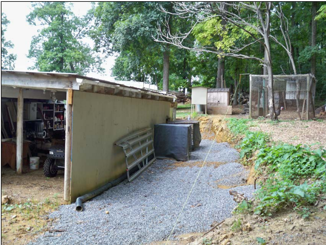
Rear of Property – String Line from Rebar
