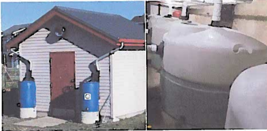
Figure 8: Rain barrels and cisterns
