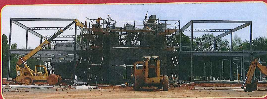
Work continues on the administrative office which will consolidate four offices in Berkeley and Jefferson counties. The office building is slated to be complete shortly after the first of the year.
