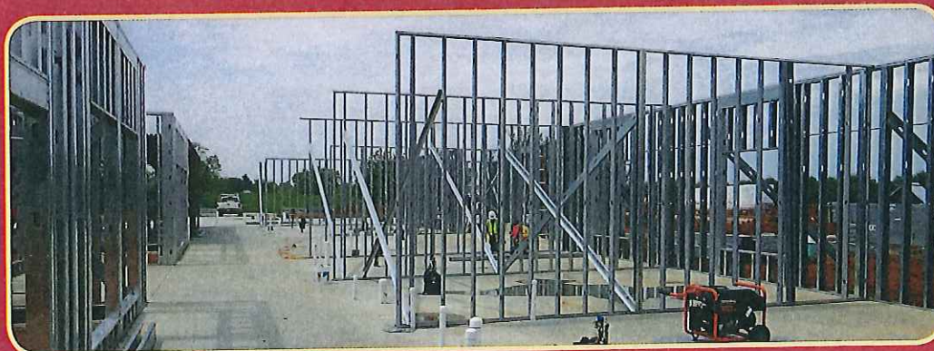
Steel support beams go up on the interior of the inpatient unit, which is slated to be complete before year's end.
