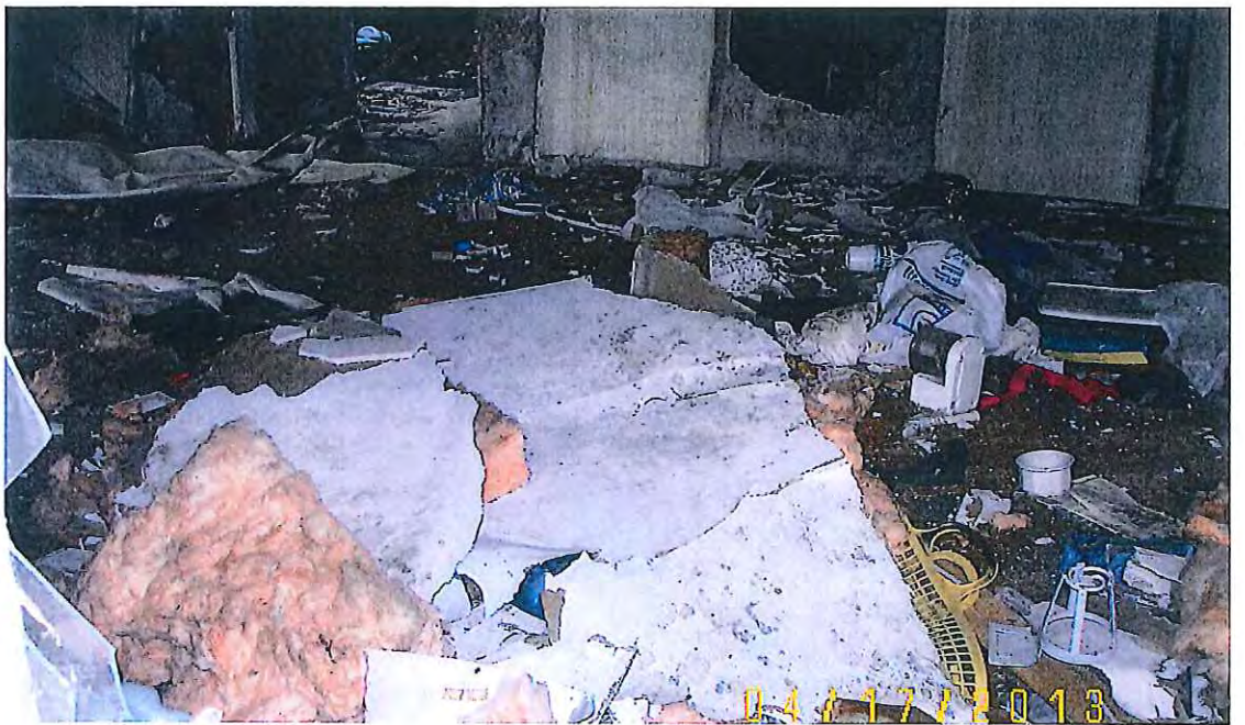
Trash, debris, black mole & vandalism in living room
