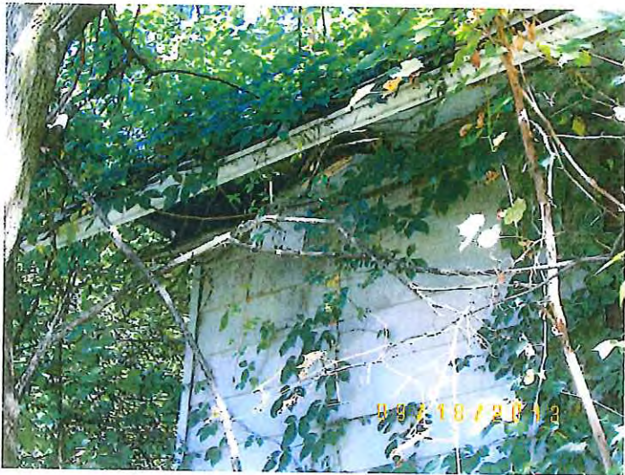
Rear soffit is decayed.
