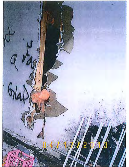
Black mold on walls
