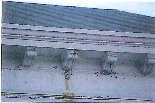
3.3.c Cornice in rear addition, metal, note rust at joint.
