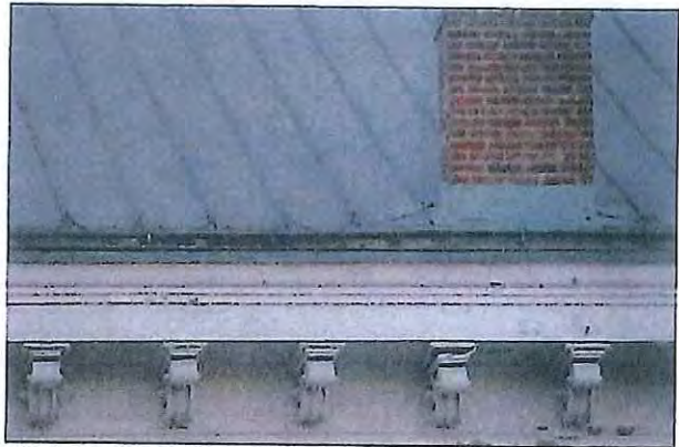
3.3.d Cornice, wood, in original section, showing location of chimney flashing, rust in liner, heating element. Note beneath this masonry is also damaged from moisture.
