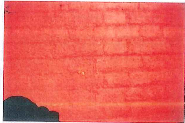
5.1.f Detail of painted brick on original section.
