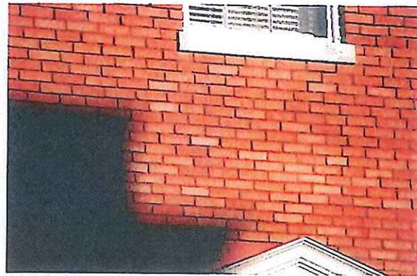
5.1.j Washed out mortar on addition wall.
