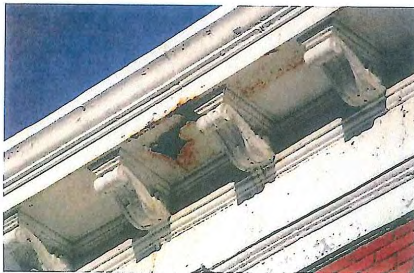
3.3.e Hole in metal soffit in addition.
