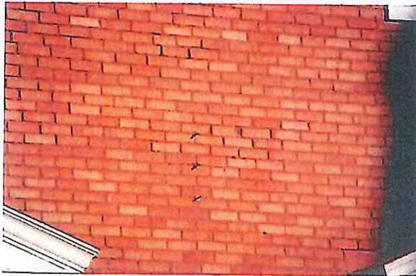
5.1.i Extraneous bracket on addition wall.
