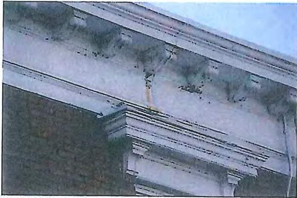
3.3.a Cornice in rear addition, metal, note rust at joint.
