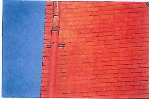
5.1.h Washout of mortar adjacent to downspout in addition.
