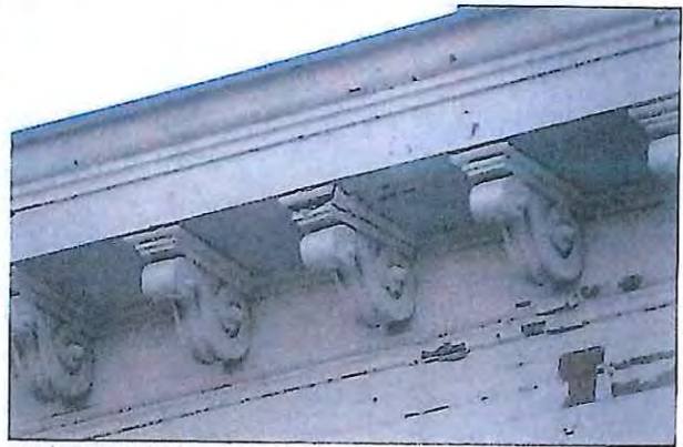
3.3.b Cornice, wood, in original section, note loose bracket and peeling paint.
