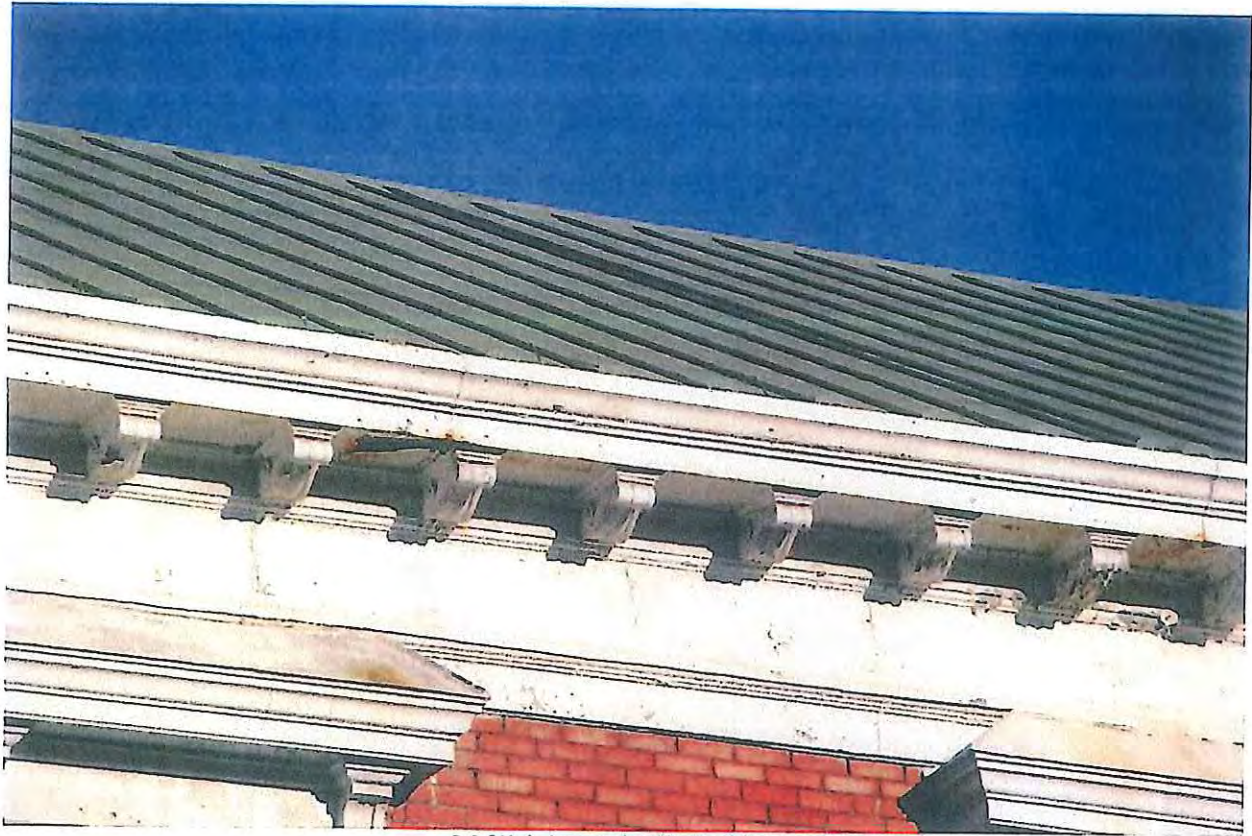
3.3.f Hole in metal soffit in addition.
