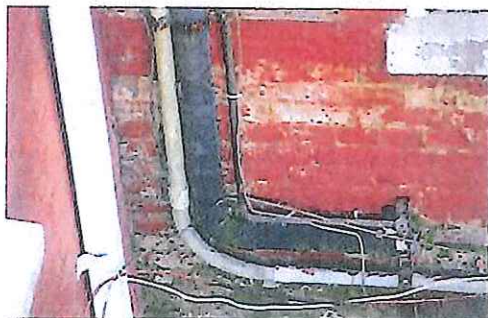
5.1.k Moisture damage to masonry on east elevation near hyphen.
